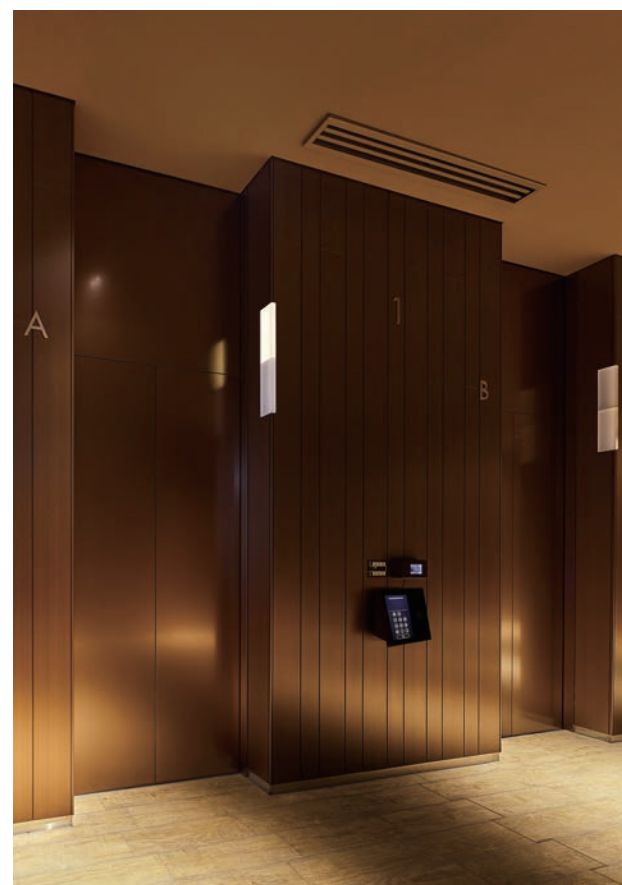
21-person passenger elevator, 1st floor
