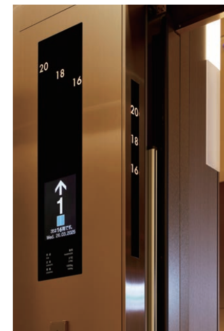
27-person passenger elevator, destination floor indicator inside car
