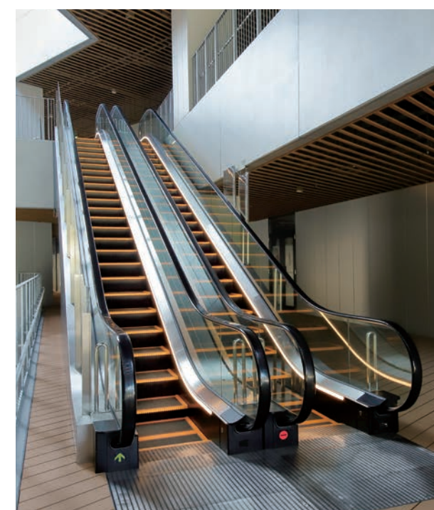
Escalator, 4th floor (Nagasaki Stadium City South)
