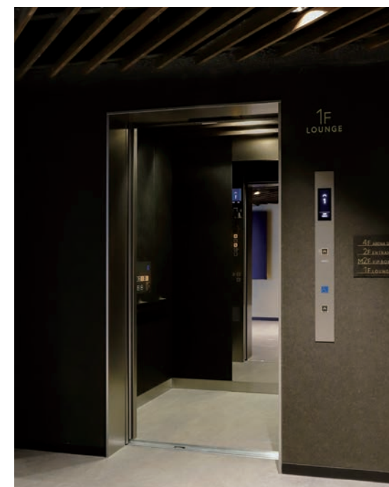
15-person passenger elevator, 1st floor (Happiness Arena)
