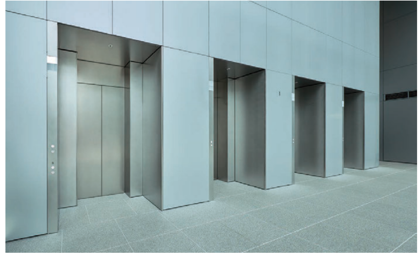
24-person passenger elevator, 1st floor
