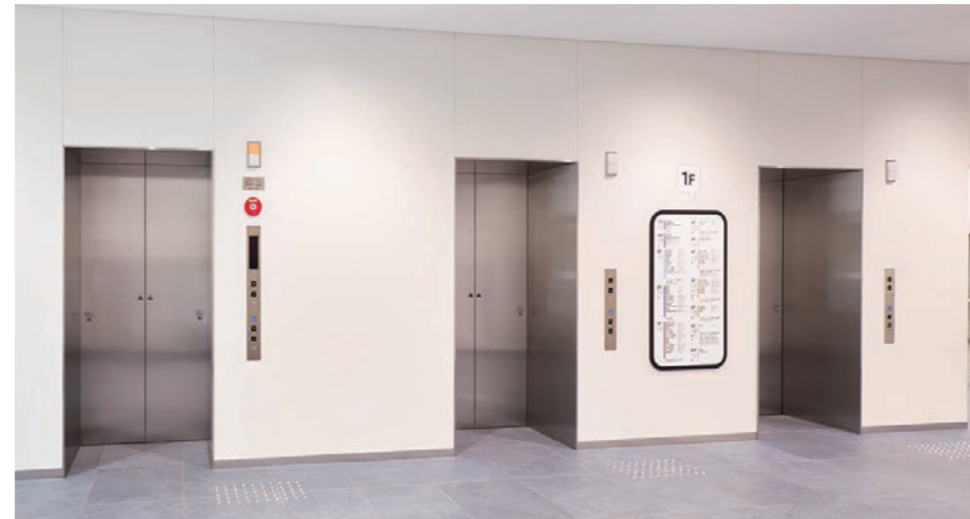
17-person passenger (emergency) elevator (for staff), 1st floor
