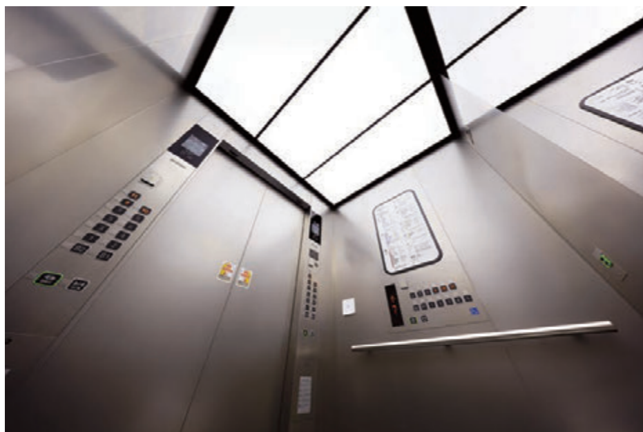
17-person passenger (emergency) elevator (for city office visitors), elevator car ceiling
