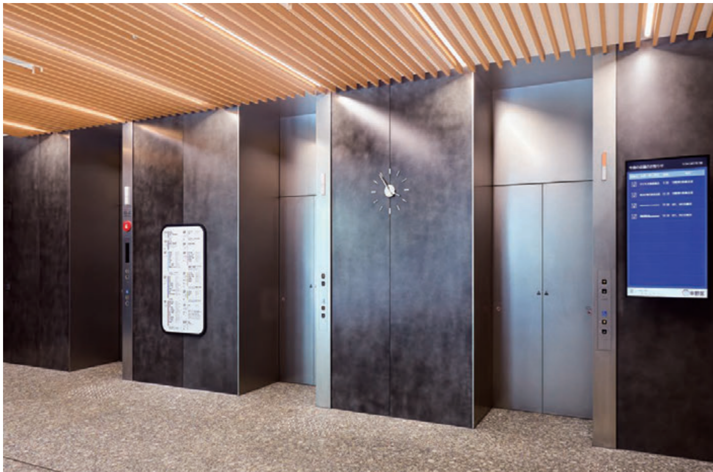
17-person passenger (emergency) elevator (for city office visitors), 1st floor
