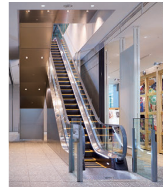
Escalator (for city office visitors), 1st floor
