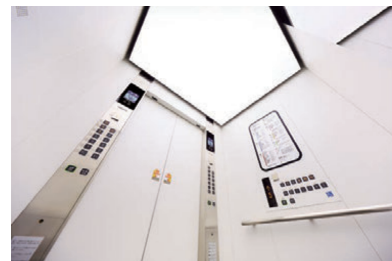
17-person passenger elevator (for staff), elevator car ceiling
