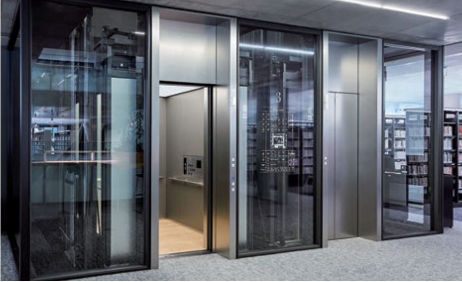
20-person passenger (observation) elevator, 3rd floor
