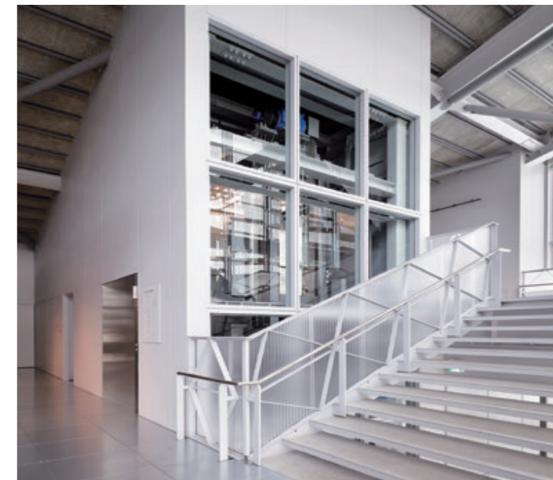
18-person passenger and freight (observation) elevator, elevator shaft (NOVARE Academy)
