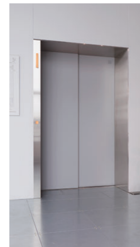
18-person passenger and freight (observation) elevator, 2nd floor (NOVARE Academy)
