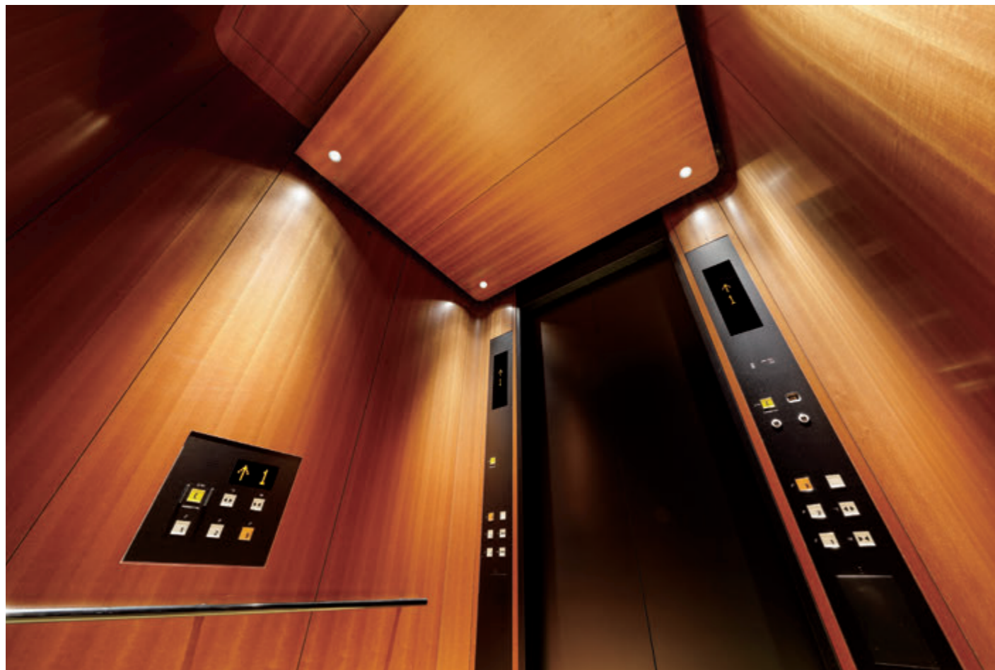
26-person passenger and freight (and emergency) elevator, elevator car ceiling (NOVARE Archives)
