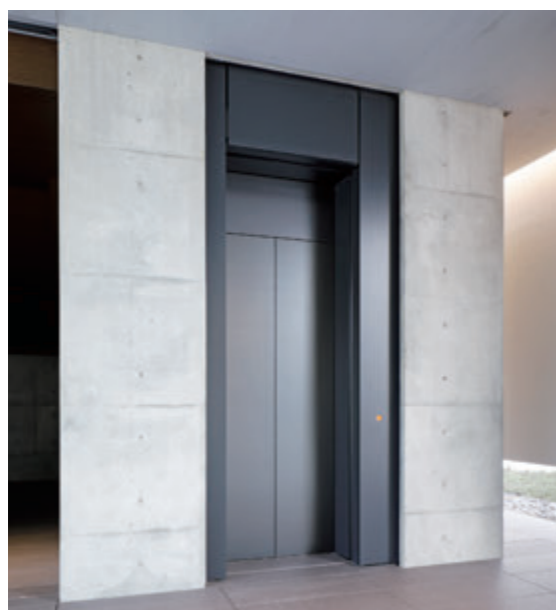
26-person passenger and freight (and emergency) elevator, 1st floor (NOVARE Archives)
