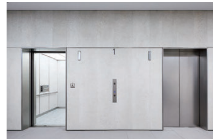
20-person passenger elevator, 1st floor, North Building
