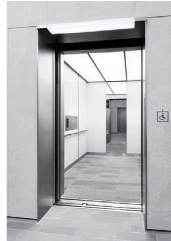
20-person passenger elevator, elevator car (1st floor, South Building)
