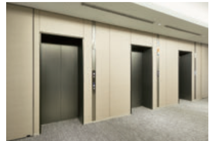
15-person passenger and freight elevator and 13-person passenger elevators, 3rd floor
