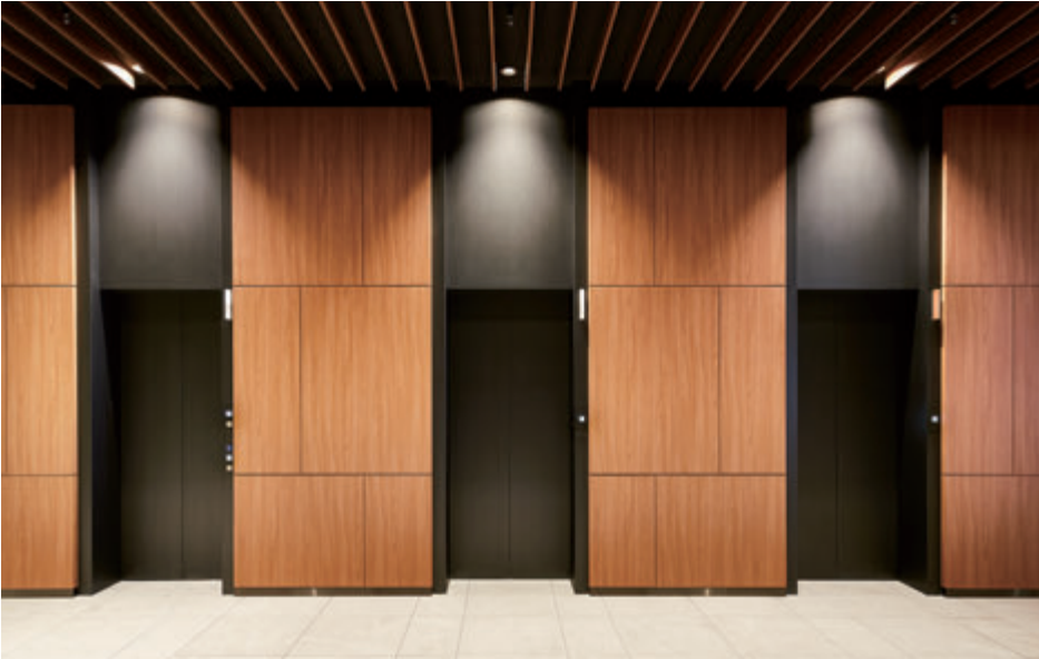
15-person passenger and freight elevator and 13-person passenger elevators, 1st floor
