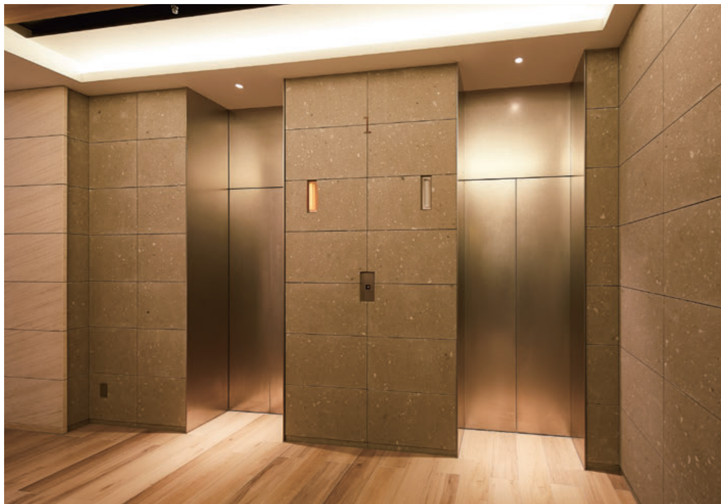
15-person passenger elevator, 1st floor
