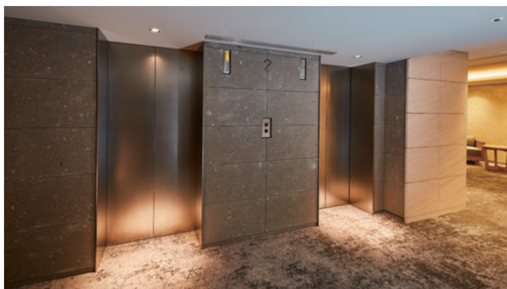
15-person passenger elevator, 2nd floor
