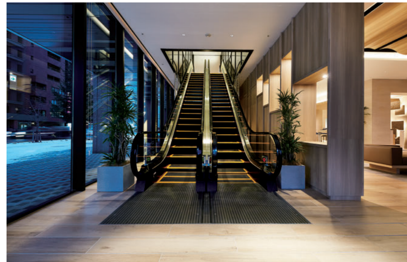
Escalator, 1st floor
