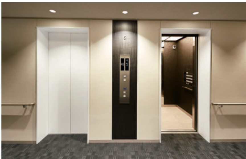
11-person passenger elevator, 5th floor (ONE Sapporo STATION Tower)
