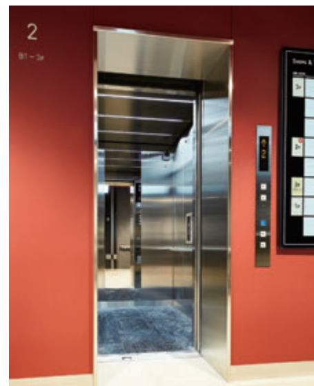
11-person passenger elevator, 2nd floor (Satsukita 8-1)
