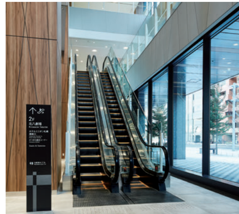
Escalator, 1st floor (Satsukita 8-1)
