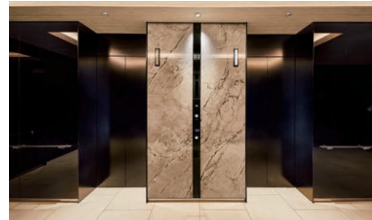
11-person passenger elevator, B1 floor (ONE Sapporo STATION Tower)
