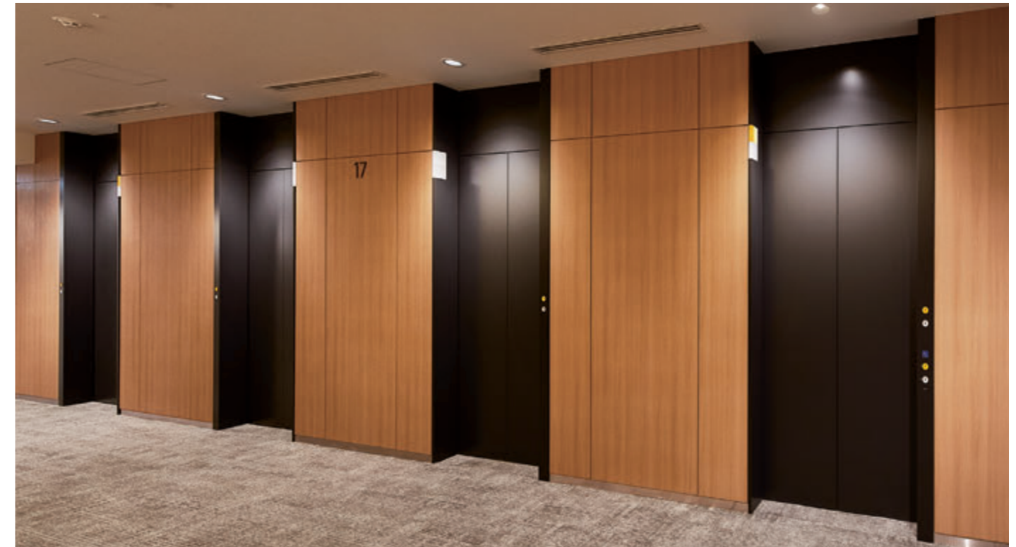
24-person passenger elevator, 17th floor
