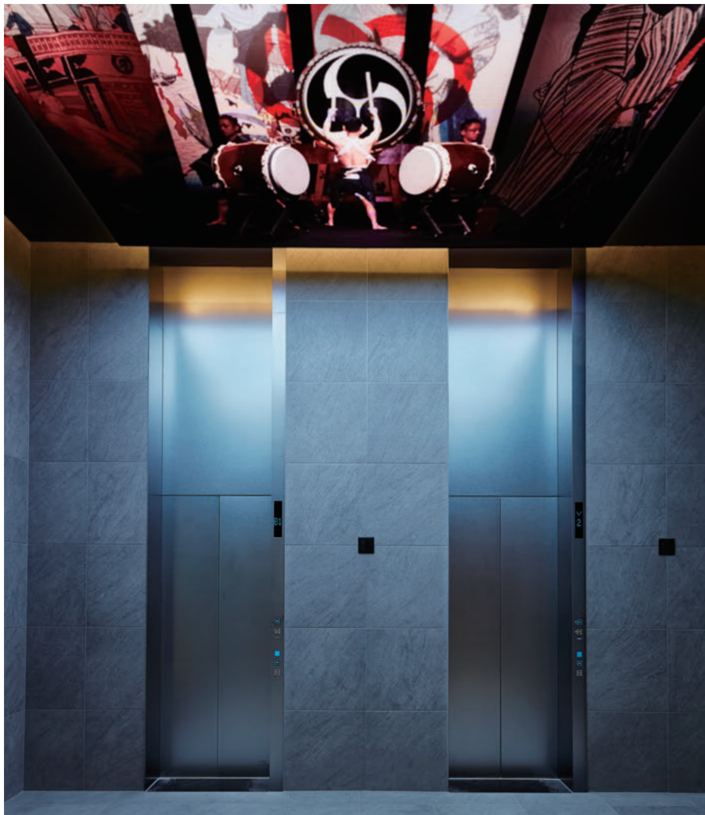
15-person passenger (observation) elevator, 2nd floor (Tokyo Toyosu Manyo Club) * Projection mapping is used on the elevator car ceiling
