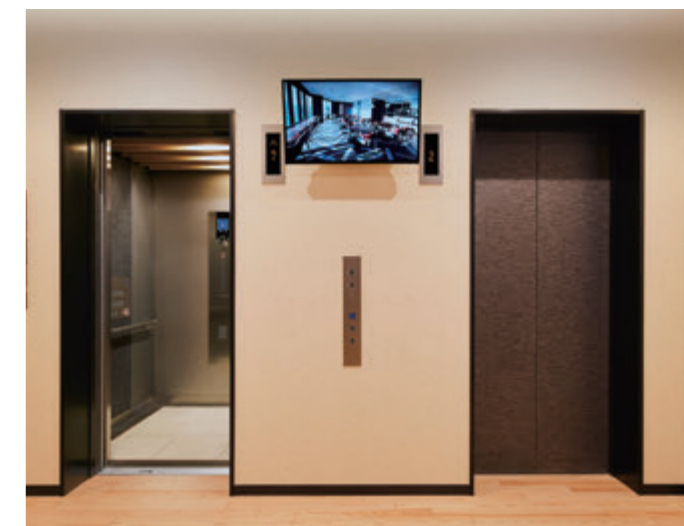
15-person passenger elevator, 7th floor (Tokyo Toyosu Manyo Club)
