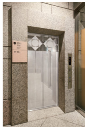
15-person passenger elevator, 2nd floor (after renovation)
