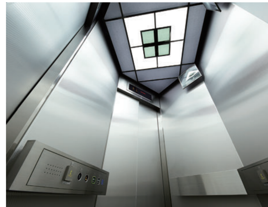
11-person passenger elevator (with two doors, at right angles to each other), elevator car ceiling (new)
