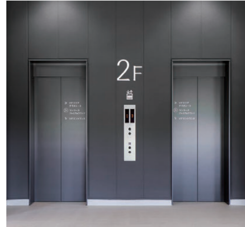
15-person passenger elevator, 2nd floor
