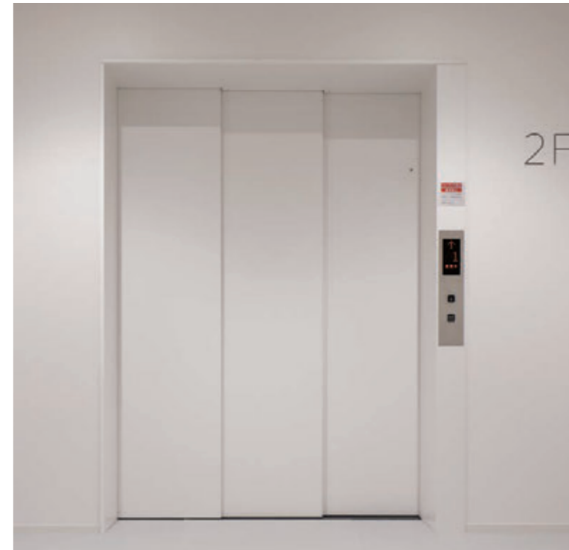
Freight elevator (2,000 kg load capacity), 2nd floor
