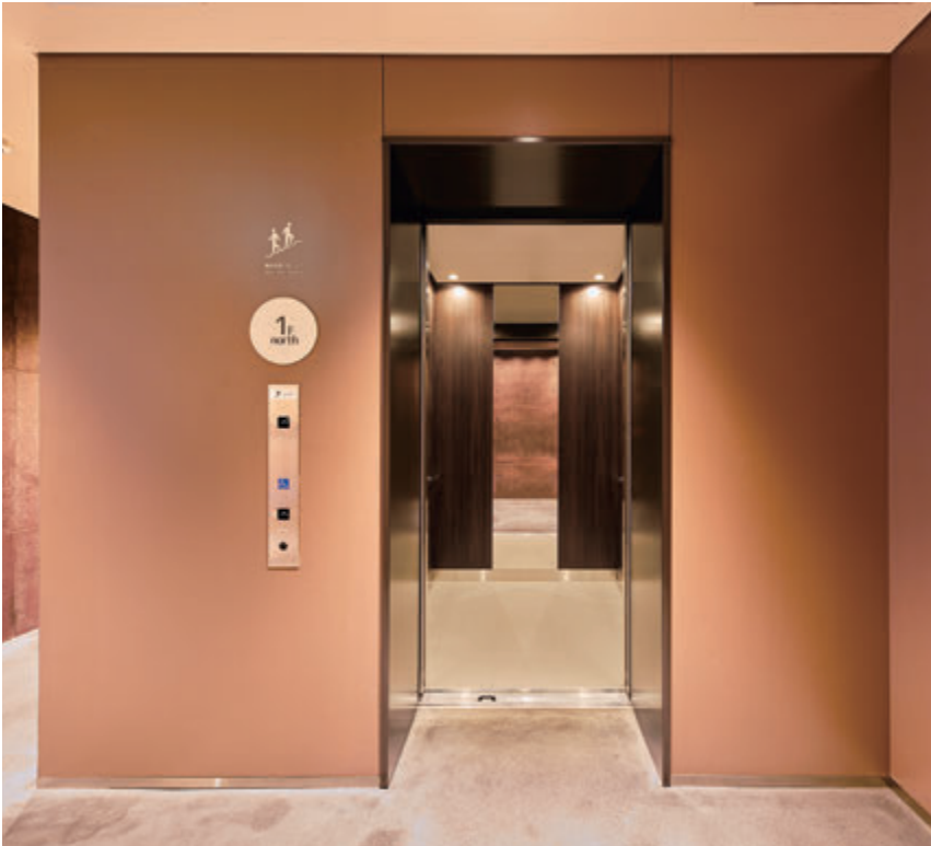
11-person passenger elevator, 1st floor
