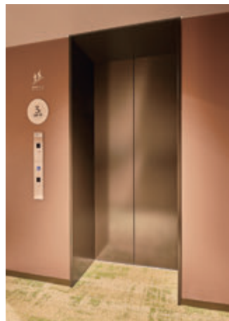
11-person passenger elevator, 3rd floor
