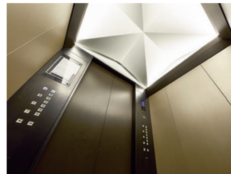
24-person passenger elevator, elevator car ceiling (S Wing upper floor elevator bank, after renovation)
