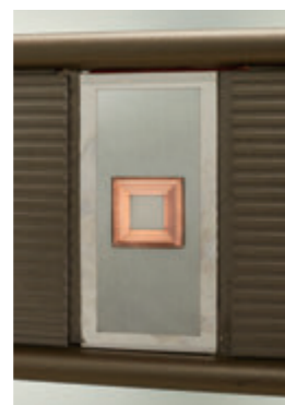
24-person passenger elevator, hall button (before renovation)
