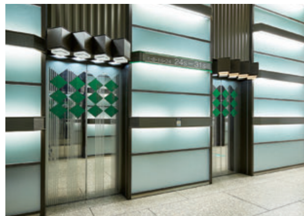
24-person passenger elevator, 1st floor hall (S Wing mid-floor elevator bank, before renovation)
