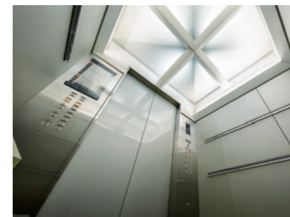
24-person passenger elevator, elevator car ceiling (S Wing mid-floor elevator bank, before renovation)
