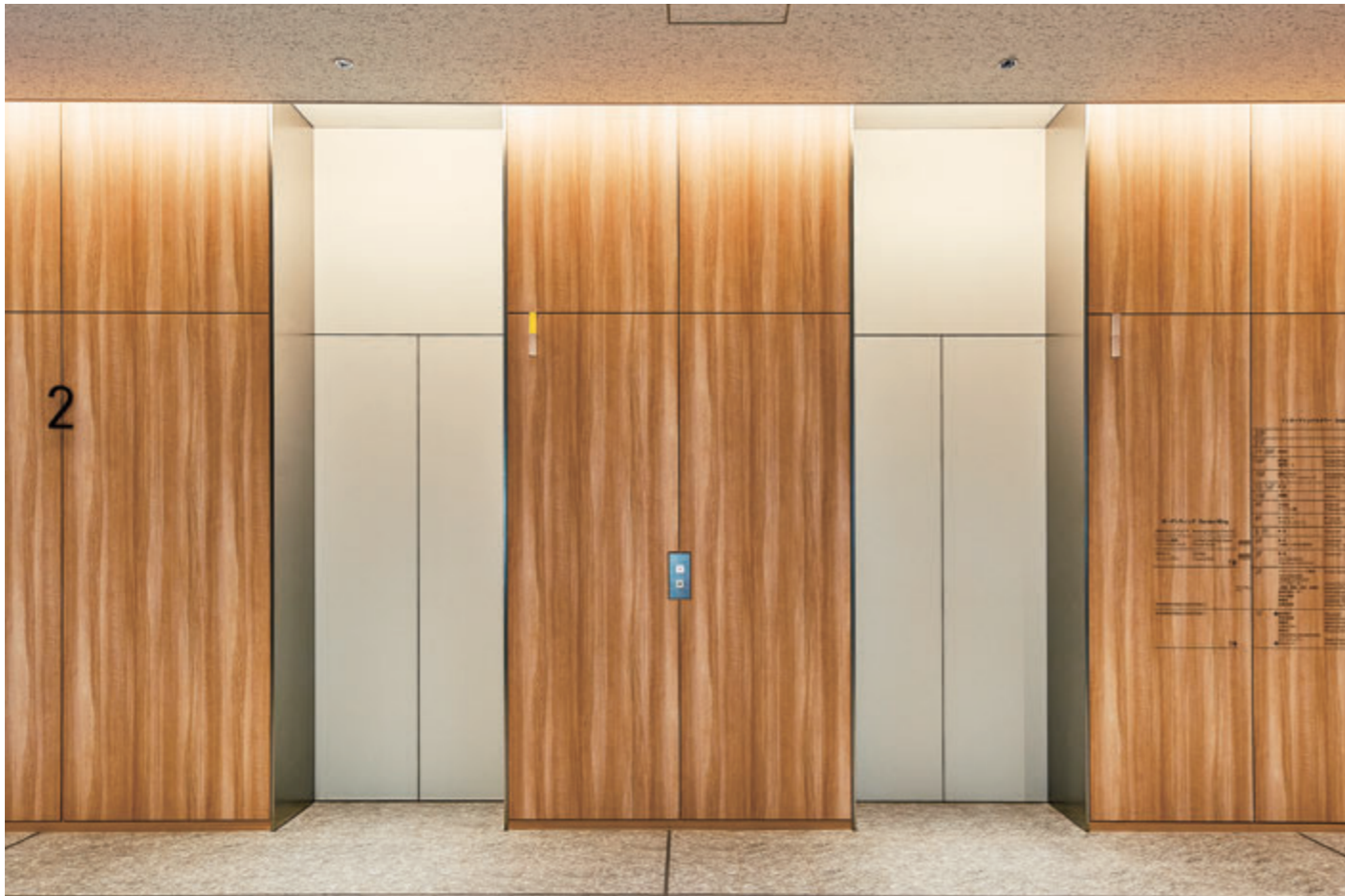
30-person passenger elevator, 2nd floor
