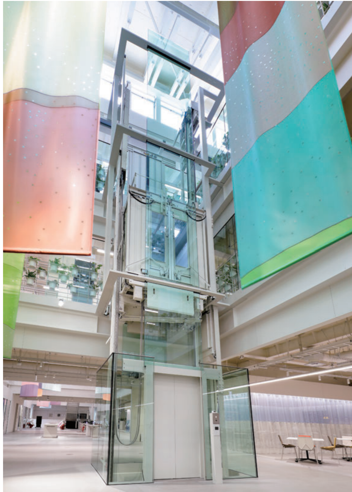
24-person passenger elevator, elevator shaft
