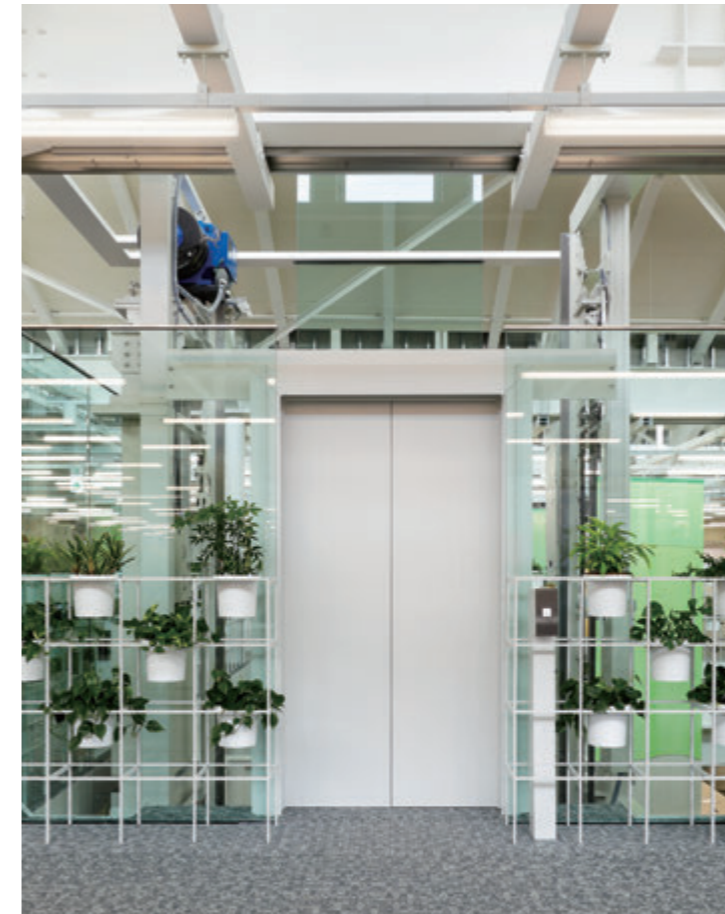
24-person passenger elevator, 3rd floor
