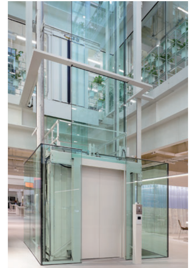
24-person passenger elevator, 1rd floor
