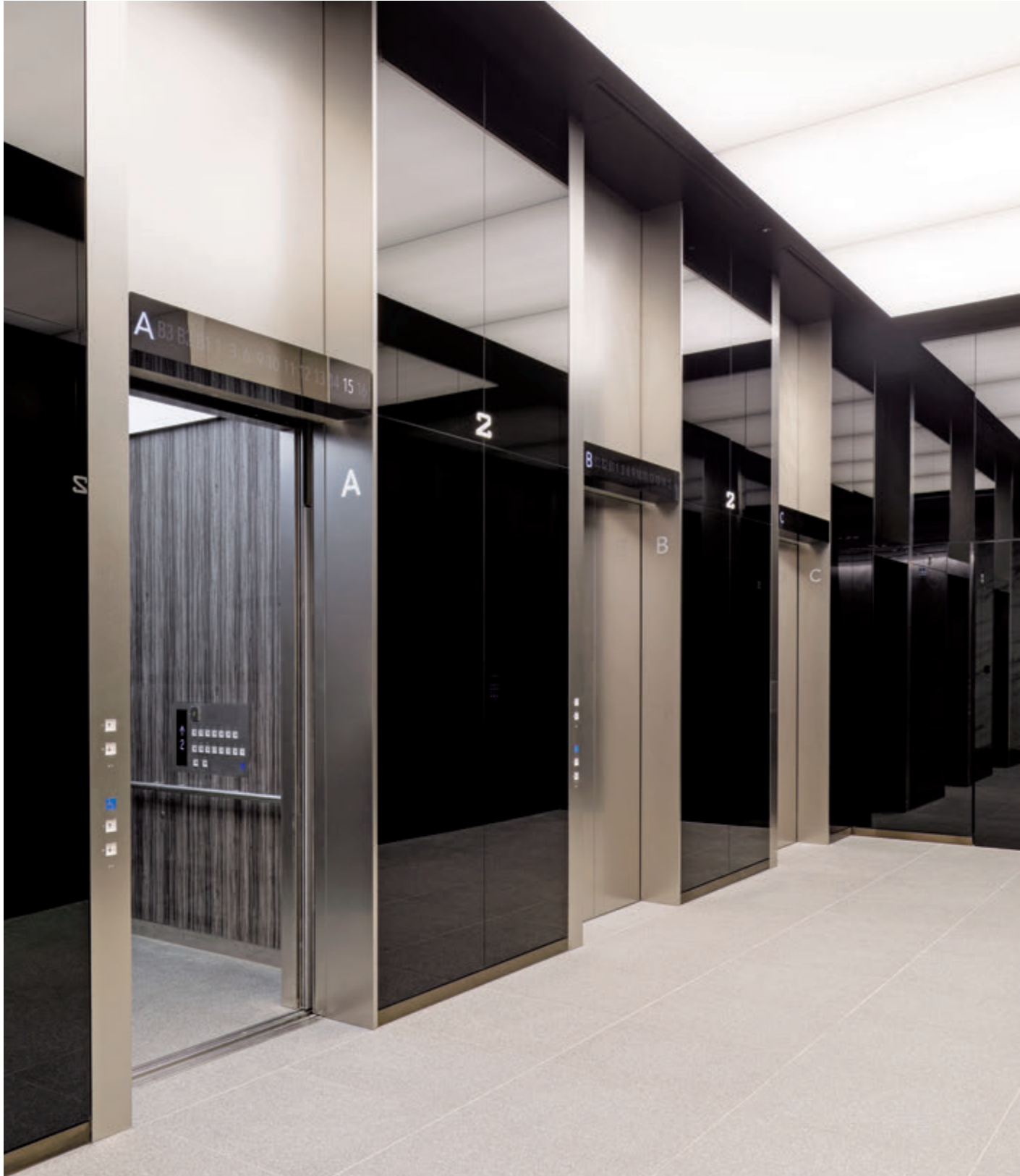
24-person passenger elevator, 2nd floor
