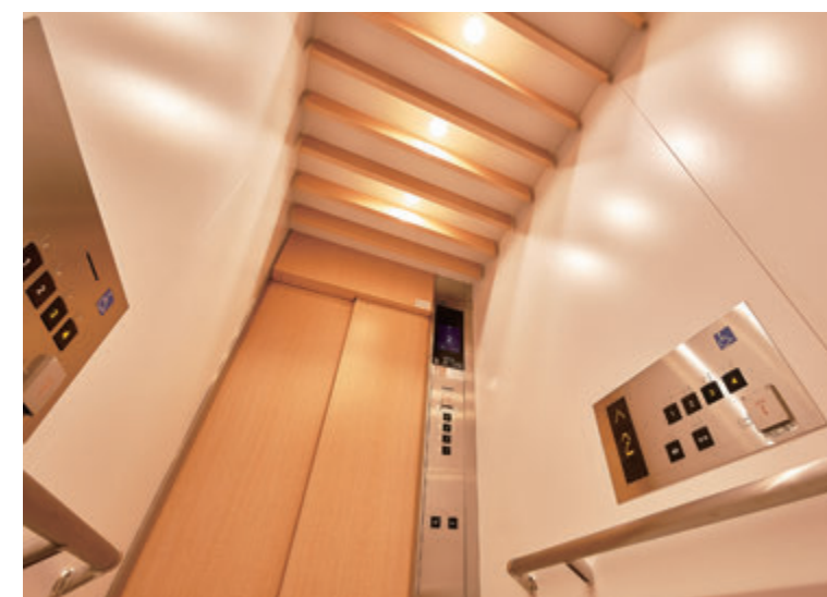
13-person passenger elevator, elevator car ceiling
