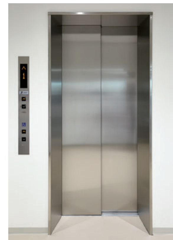
13-person passenger elevator, 3rd floor hall
