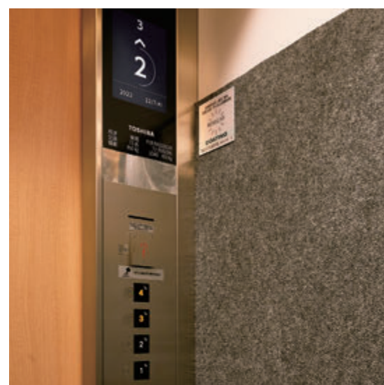
Contact-free buttons and odor, germ, and virus-resistant elevator mats made with photocatalytic material are used to improve elevator hygiene
