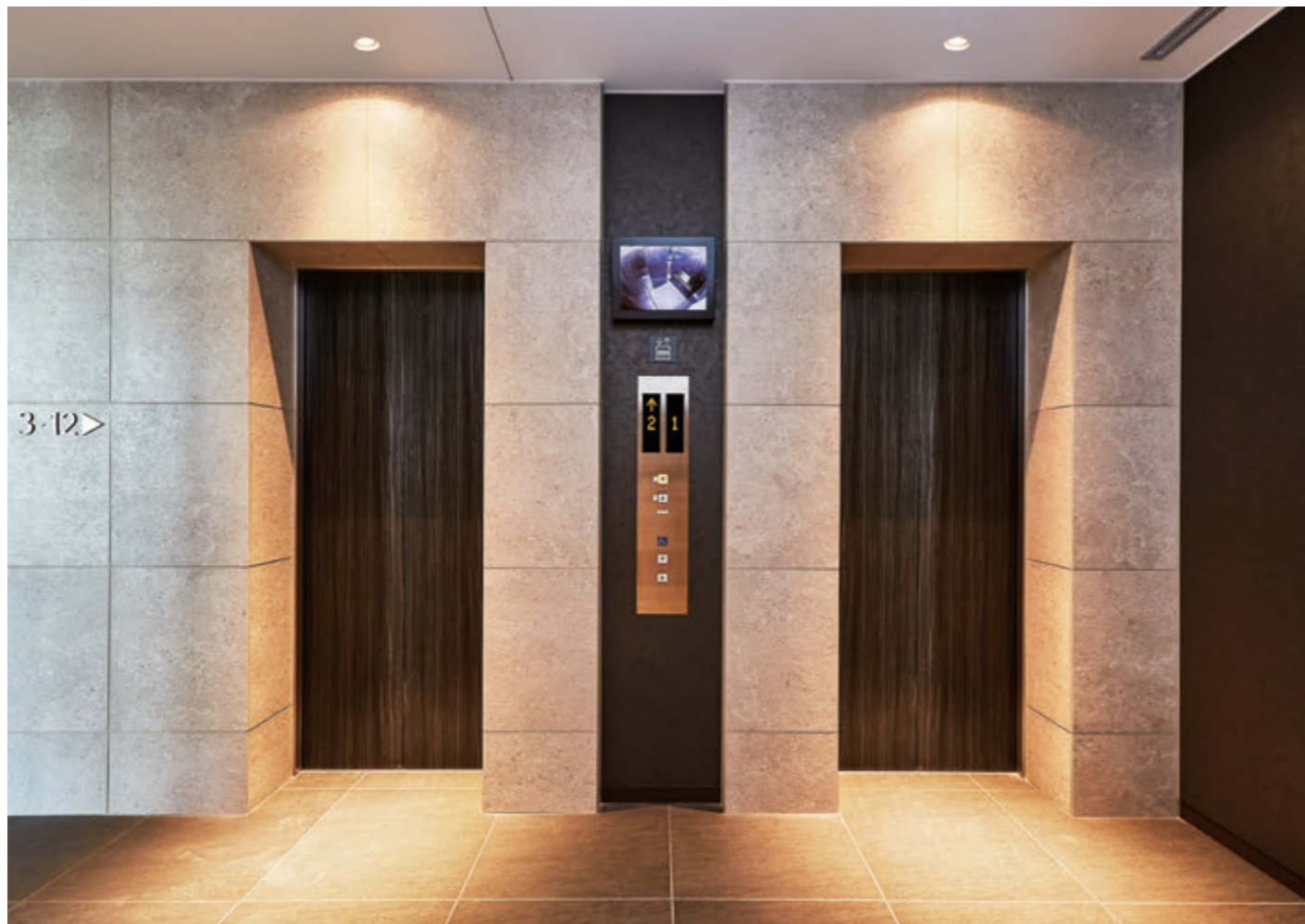
11-person passenger elevator, 1st floor hall
