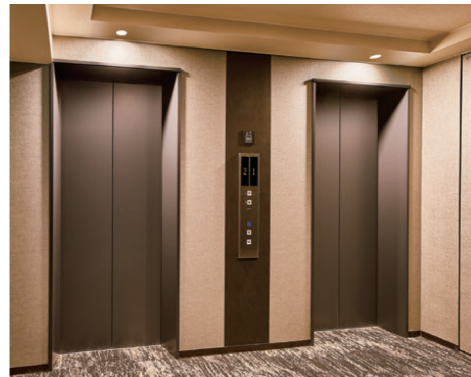
11-person passenger elevator, 2nd floor hall
