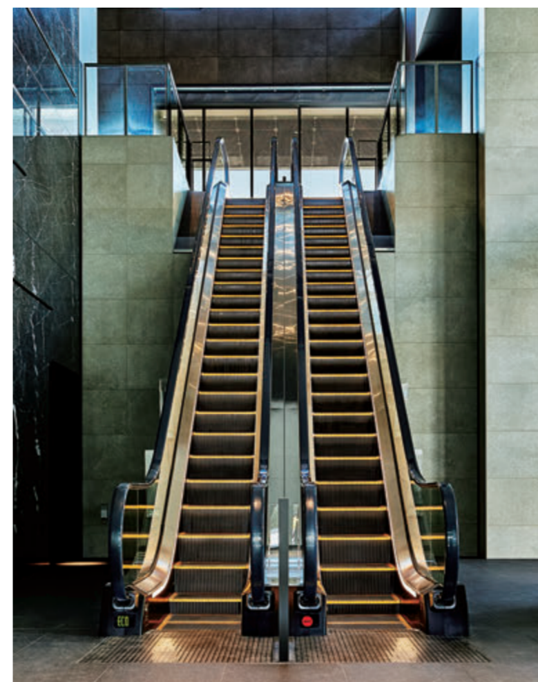
Escalator, 1st floor
