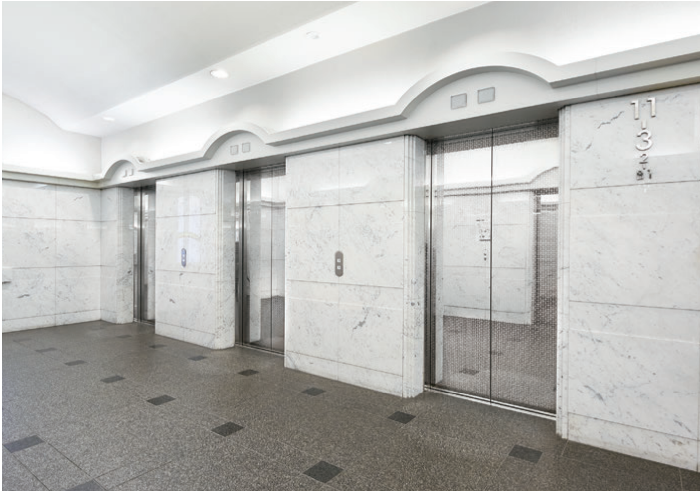
20-person passenger elevator, 1st floor hall (after renovation)
