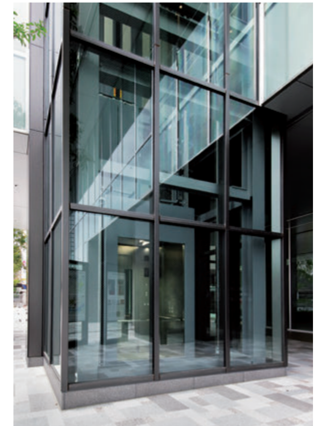
15-person passenger (observation) elevator, 1st floor elevator shaft
