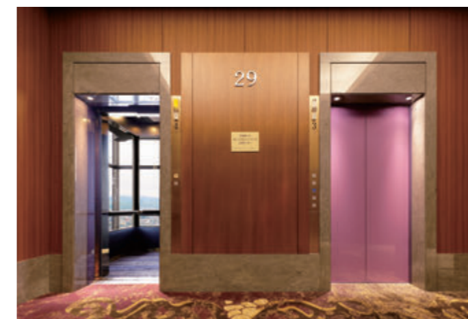
15-person passenger (observation) elevator (left)/ 20-person passenger elevator (right) 29th floor hall (after renovation)
