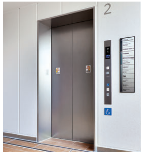
15-person passenger elevator, 2nd floor landing
