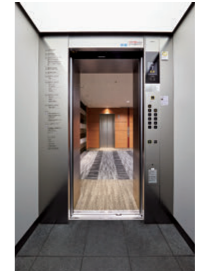
15-person passenger elevator, elevator car (Furumachi Rufuru)
