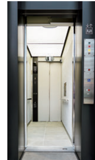
13-person passenger elevator, elevator car (Furumachi Rufuru Plaza)
