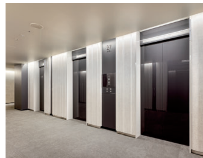
24-person passenger elevator, 27th floor landing
