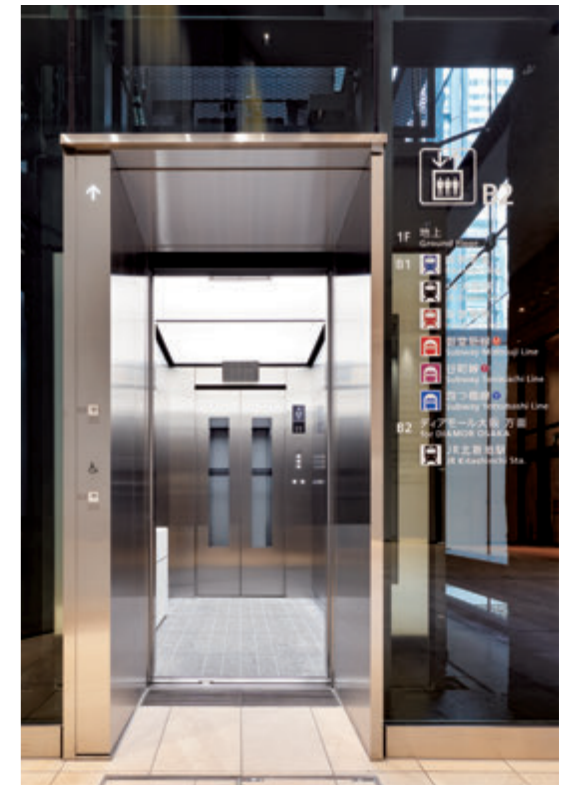
20-person passenger elevator, B2 floor landing
