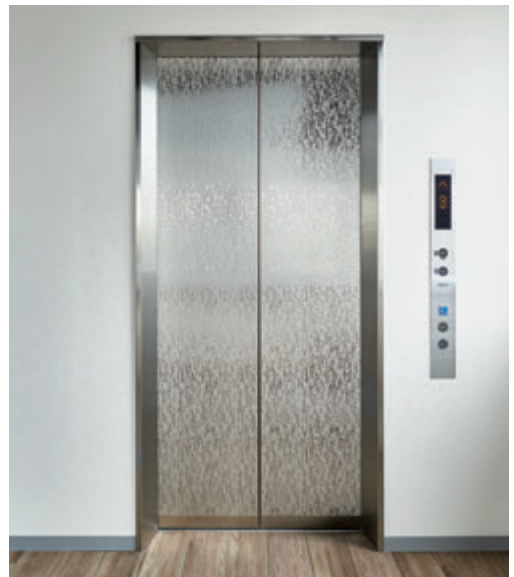
15-person passenger elevator, 3rd floor
