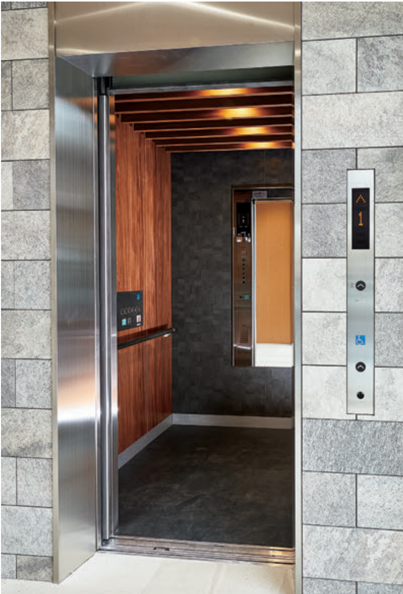
15-person passenger elevator, 1st floor
