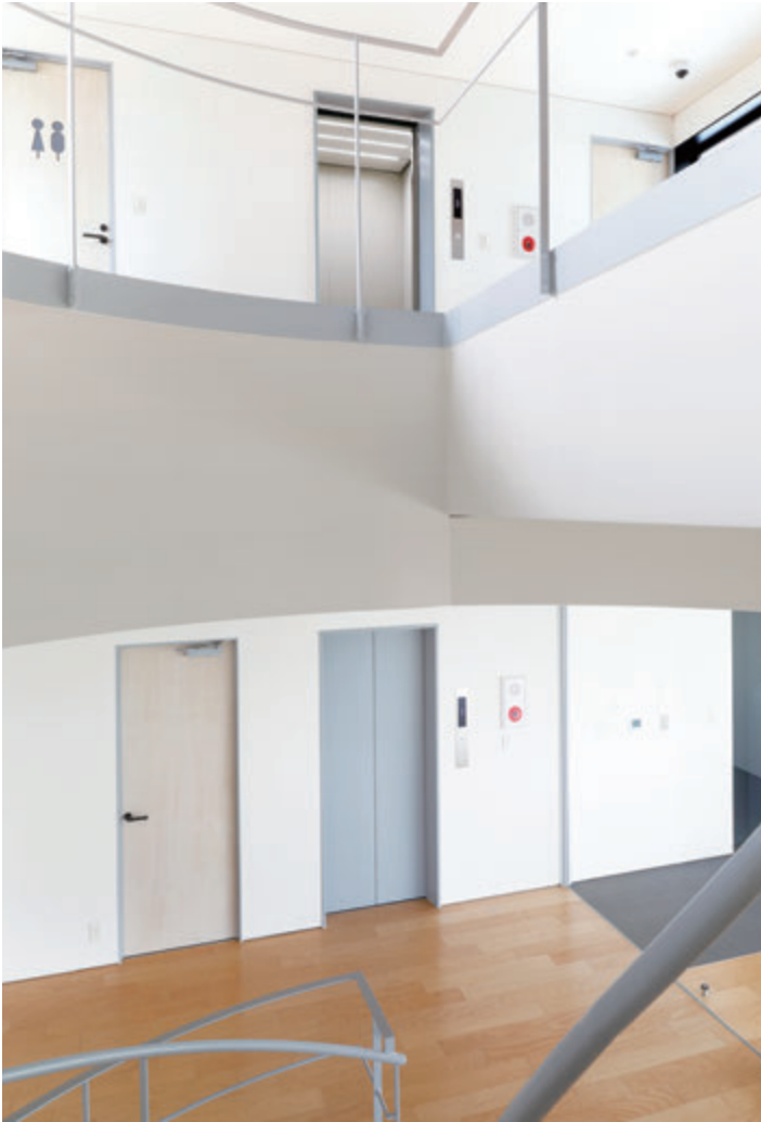
9-person passenger elevator, 3rd/4th floors
