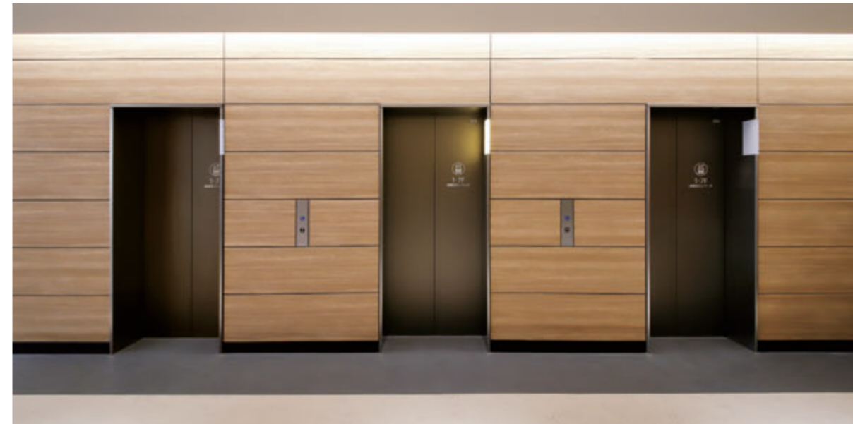
15-person passenger elevator, 1st floor hall
