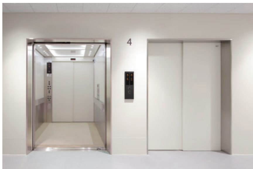
17-person passenger hospital bed elevator, 4th floor landing and car
