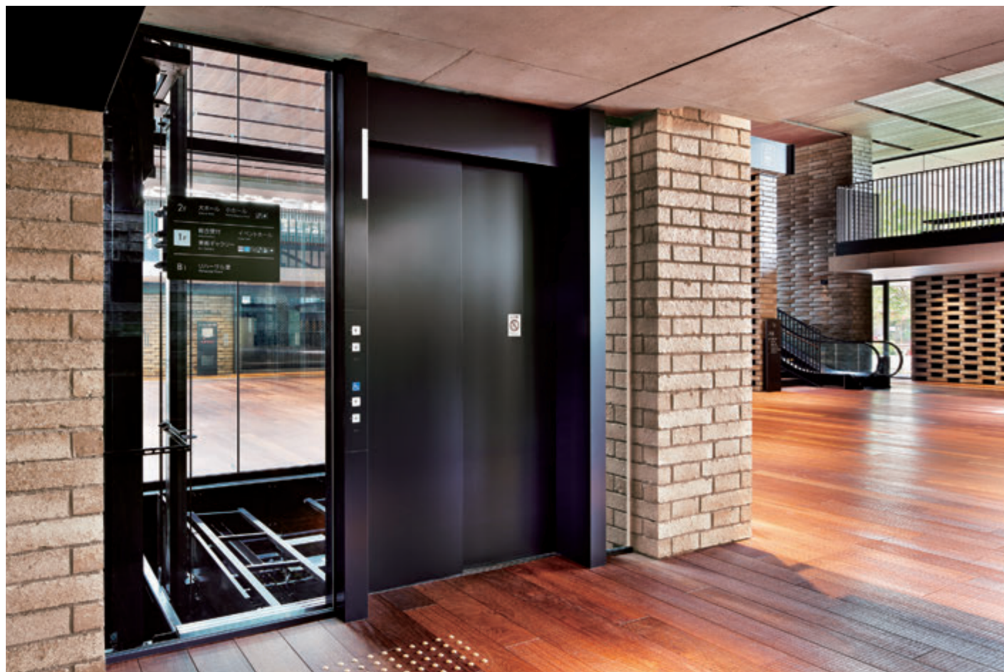
26-person passenger (observation) elevator, 1st floor lobby
