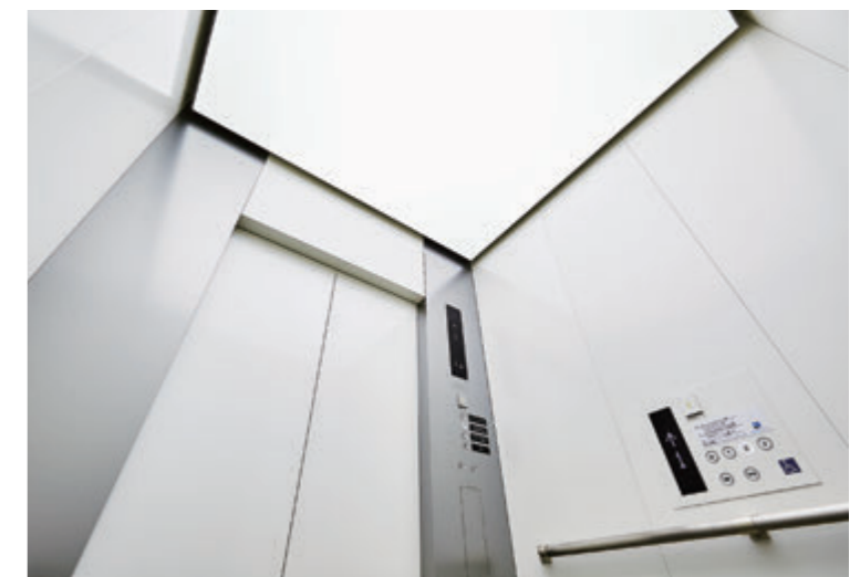
27-person passenger elevator, elevator car ceiling (elevator for Station Conference Kawasaki)
