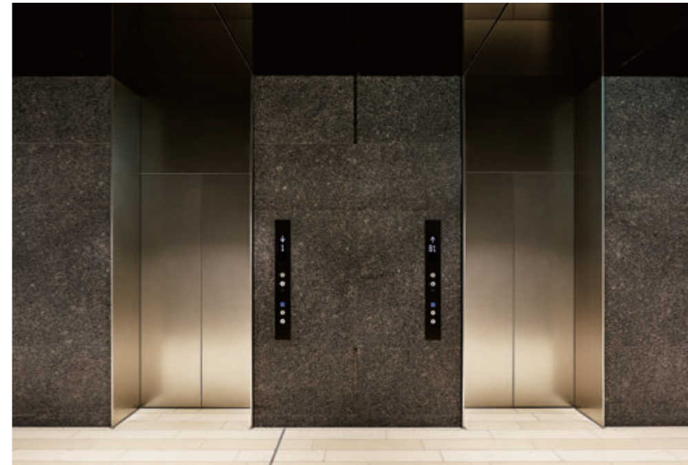
27-person passenger elevator, 2nd floor hall (elevator for Station Conference Kawasaki)
