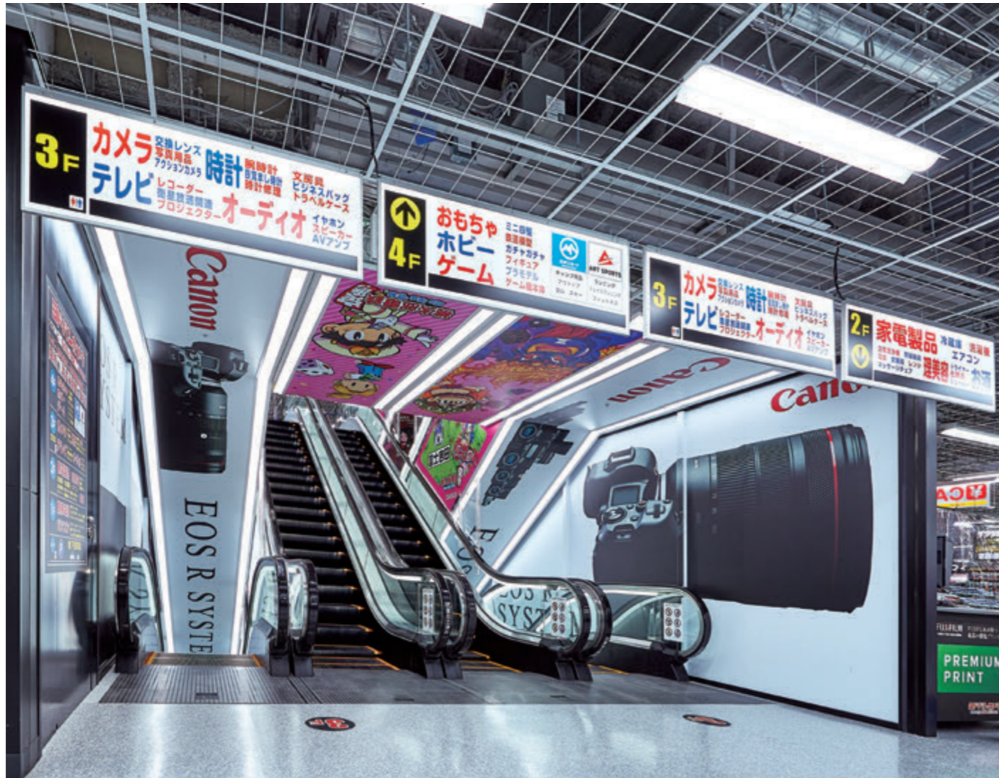
Escalator, 3rd floor landing
