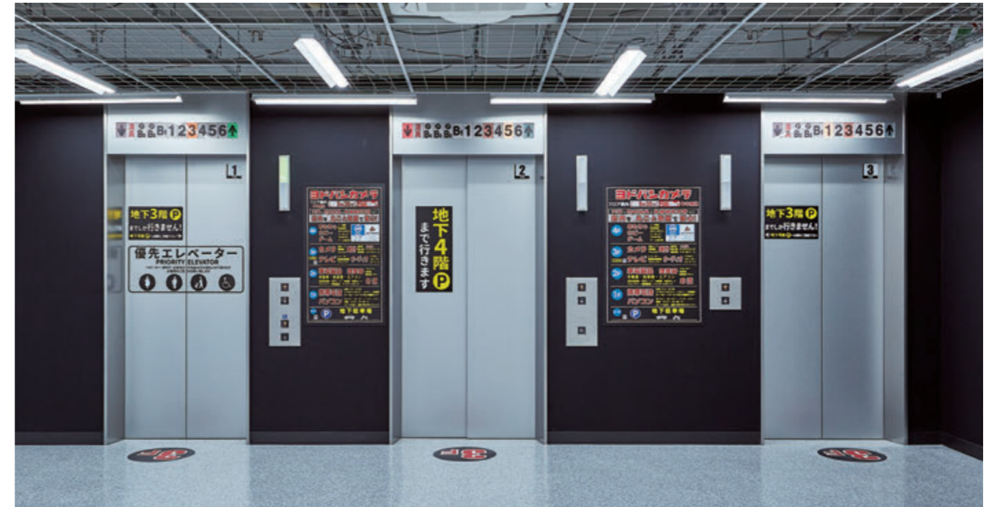
24-person passenger elevator, 3rd floor elevator hall
