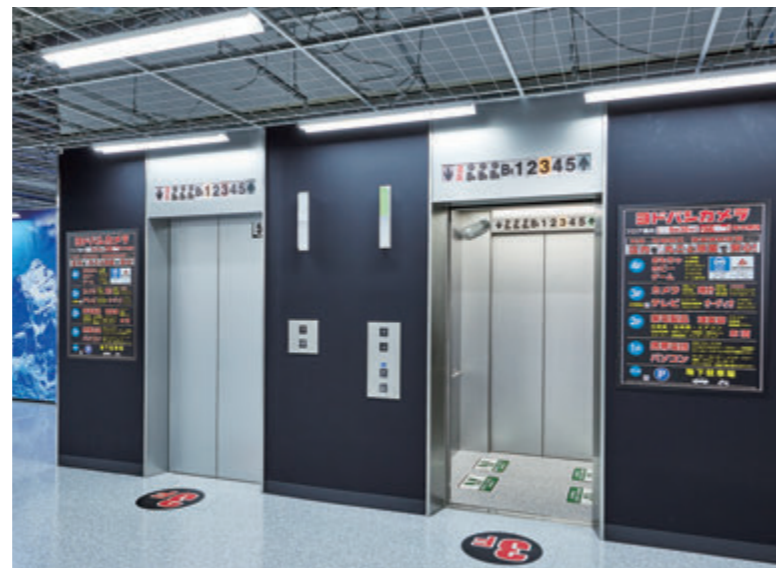
15-person passenger elevator, 3rd floor elevator hall
