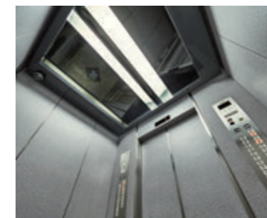
24-person passenger elevator car ceiling (before renewal)
