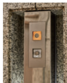
Elevator hall buttons, 1st floor (before renewal)
