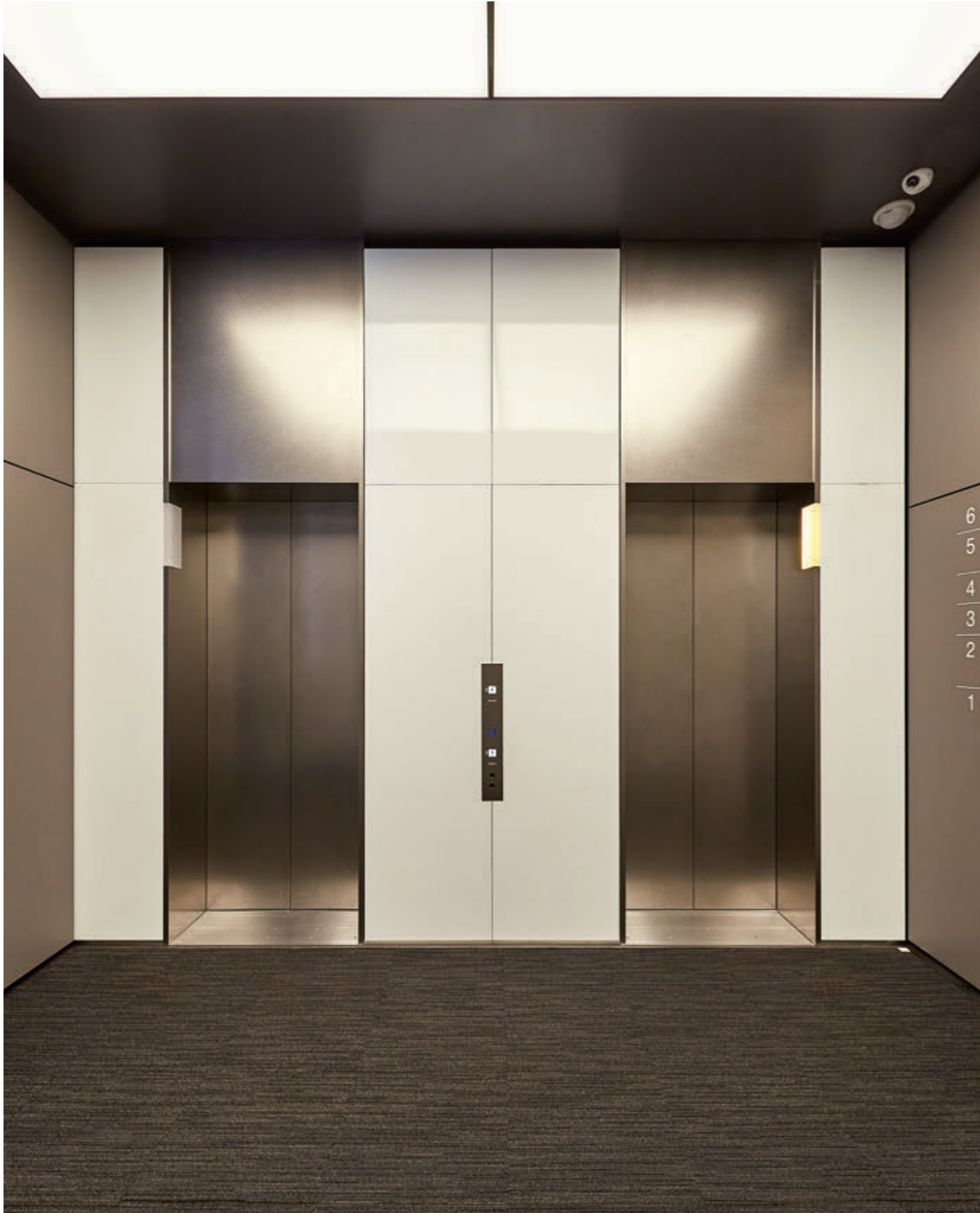
15-person passenger elevator, 1st floor elevator hall
