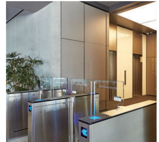
15-person passenger elevator, view from 1st floor lobby
