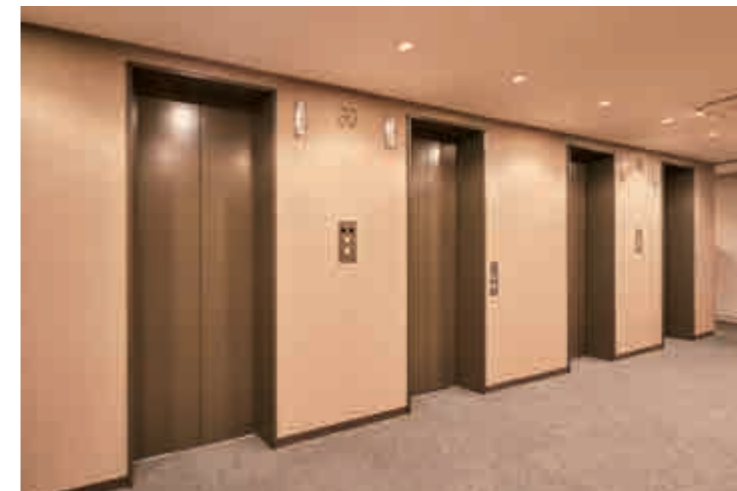
11-person passenger elevator, 30th floor elevator hall
