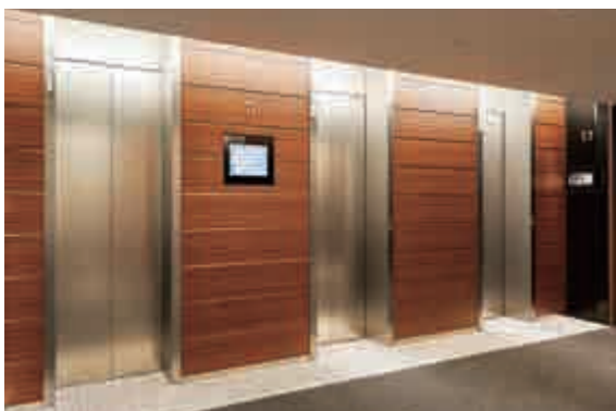
30-person passenger elevator, 11th floor elevator hall (Mitsui Bussan Building)
