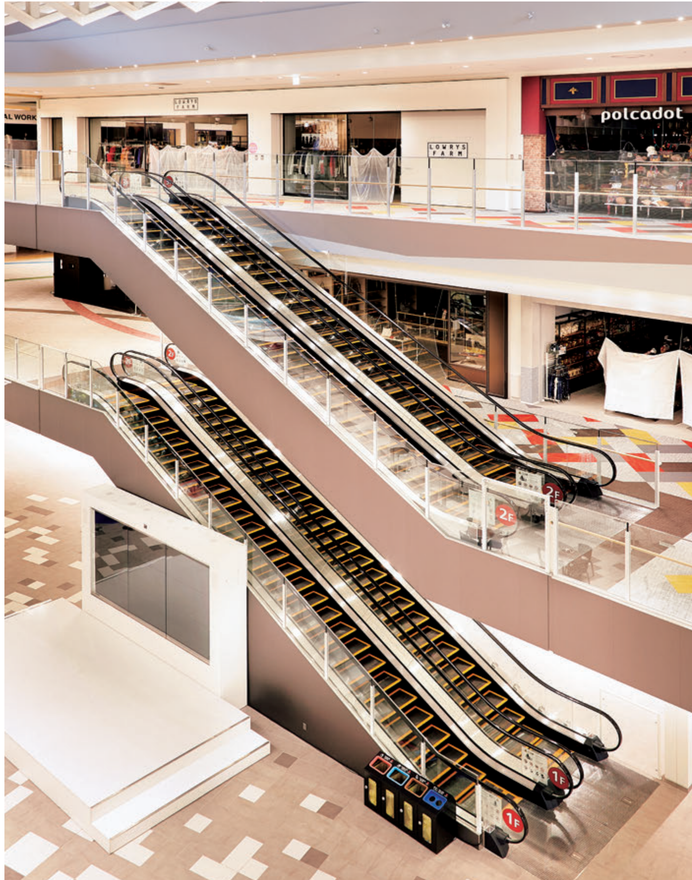
Escalator (Center Court)
