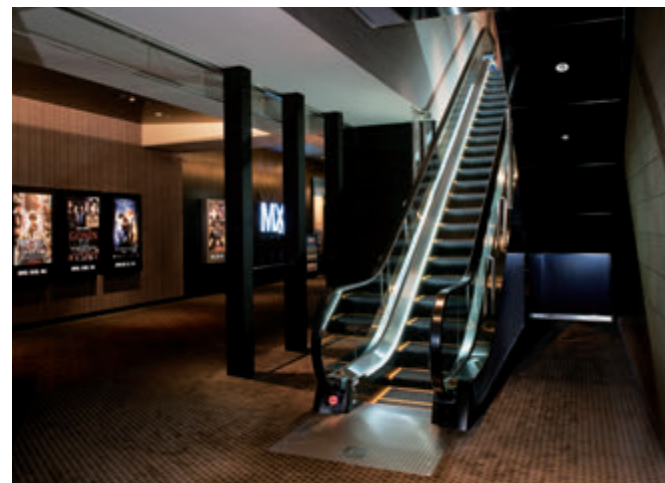
Escalator, 3rd floor landing (TOHO Cinemas Shinjuku)
