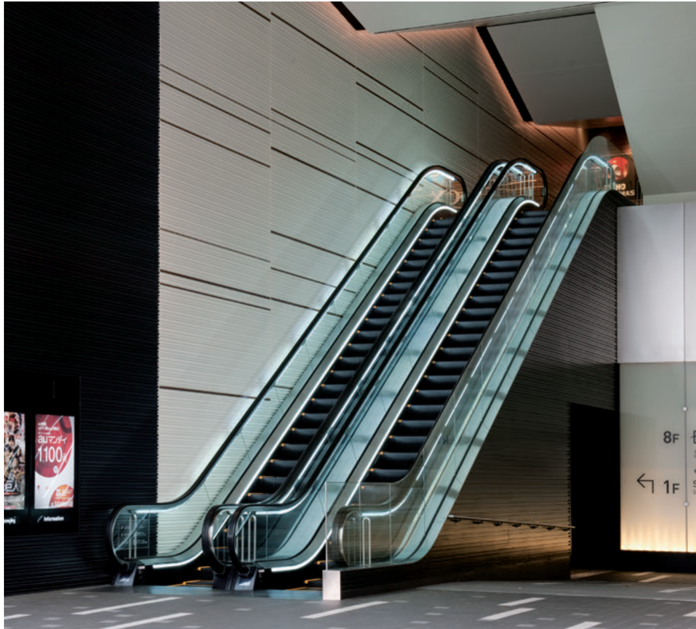
Escalator entrance (TOHO Cinemas Shinjuku)
