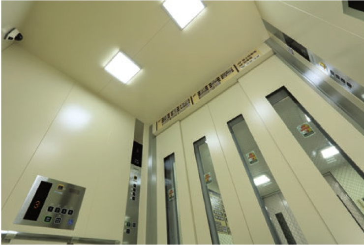
30-person passenger elevator car ceiling
