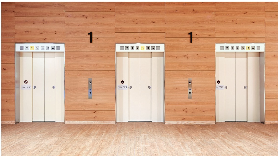
24-person passenger elevator, 1st floor hall
