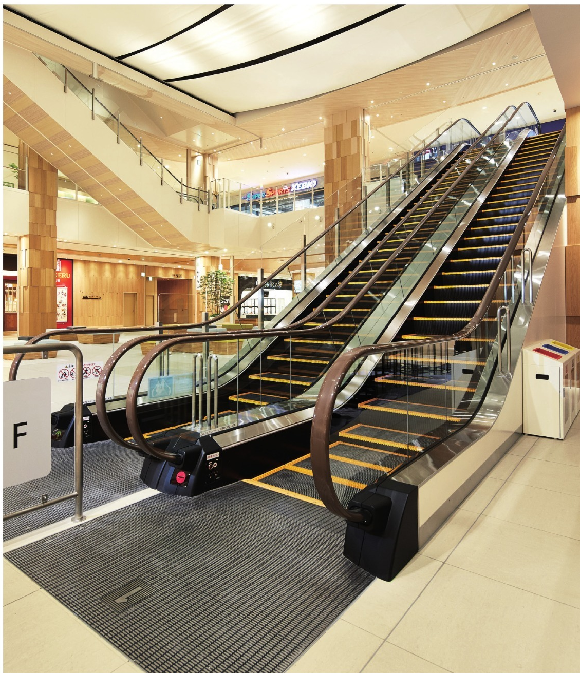
Escalator, 1st floor landing (Soyokaze Plaza)
