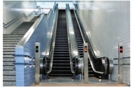
Escalator (Yagiyama Zoological Park Station, East 1 Exit)
