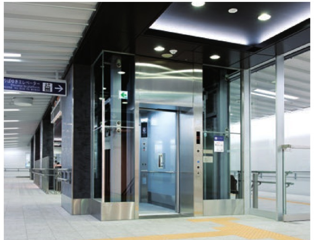
13-person passenger elevator (Omachi Nishi-koen Station, ticket gate floor)
